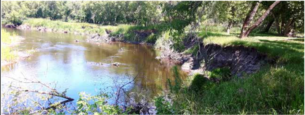
(Shoreline severely degraded by water erosion - Sturgis Regional Park)
