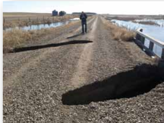
"Sleepy's Bridge" Erosion Problem (April 30/14)
