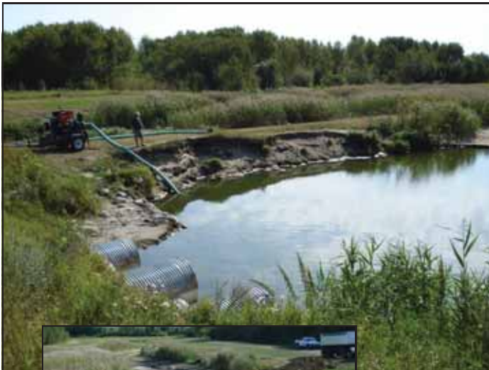
Sept. 2013 - Beginning to pump out the scour hole in preparation for infilling/construction.
